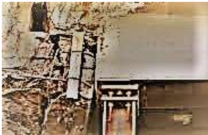
Figure 1: The problem of corrosion in the constructions.
